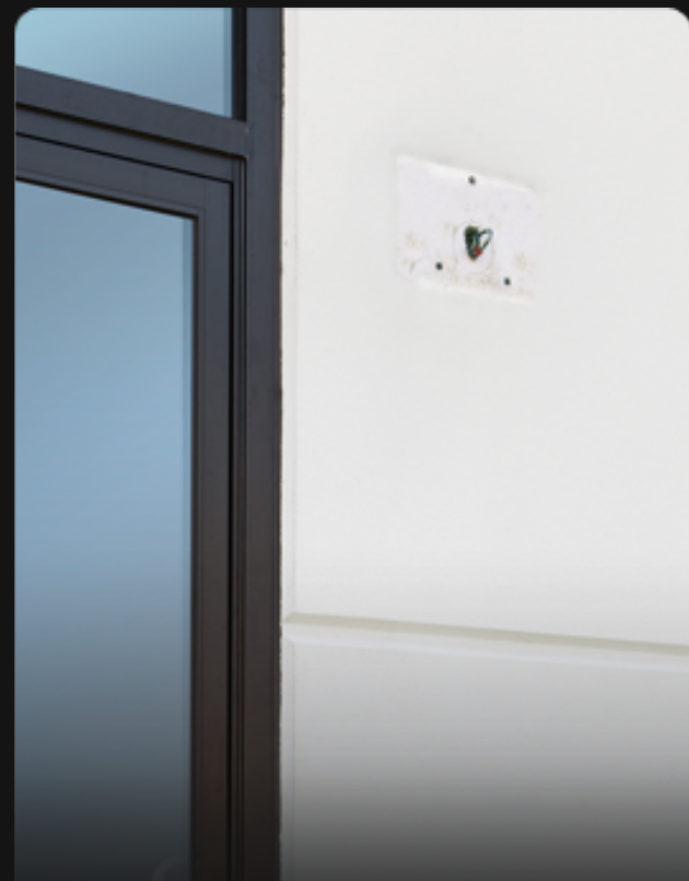
During Upgrade Wall stain left by HID wallpack
